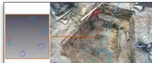
Horizontal cut of the rebars showing accurate comparison of photogrammetry to terrestrial laser scanning (TLS): blue circles represent photogrammetry, and red circles represent TLS; maximum deviation is ~6-10 millimeters.
