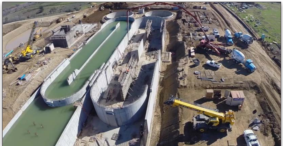
Construction of the new 13-acre, USD 48 million water recycling facility in Los Osos, California.
