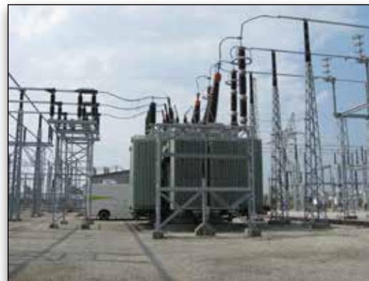
AssetWise manages the asset lifecycle of Indianapolis Power and Light Company's complex electric network.
