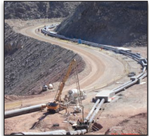
GMI SA Ingenieros Consultores developed the engineering for a permanent freshwater supply for the new concentrator process which will triple copper production.
