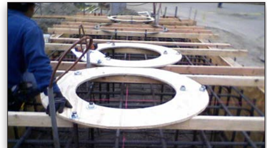
A construction crew places the vertical vessel foundation design using Bentley software.
