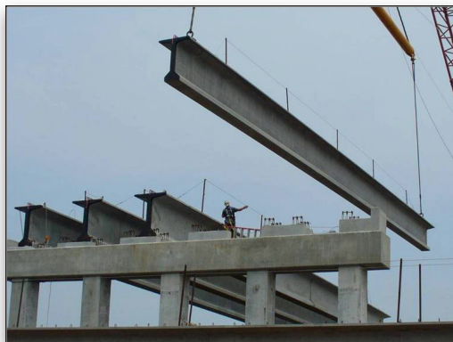
More than 345,000 linear feet of prestressed-precaster girders were designed with LEAP CONSPAN.
