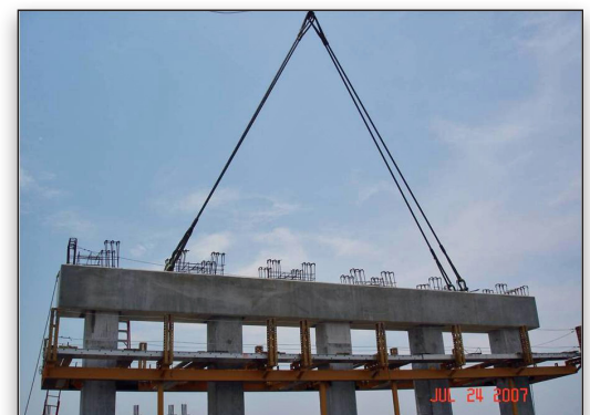
Precast reinforced concrete caps designed with LEAP RC-PIER were used for the majority of the spans.
